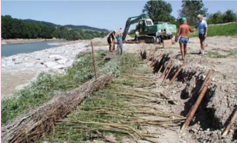
Bank protection with rip-rap of willows
