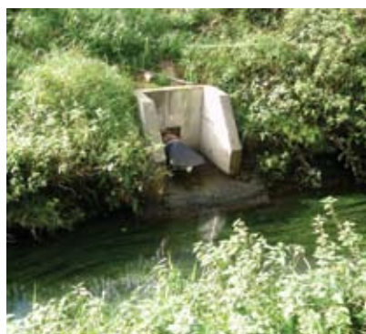
Inlet pipe into Blackwater, Mallusk
